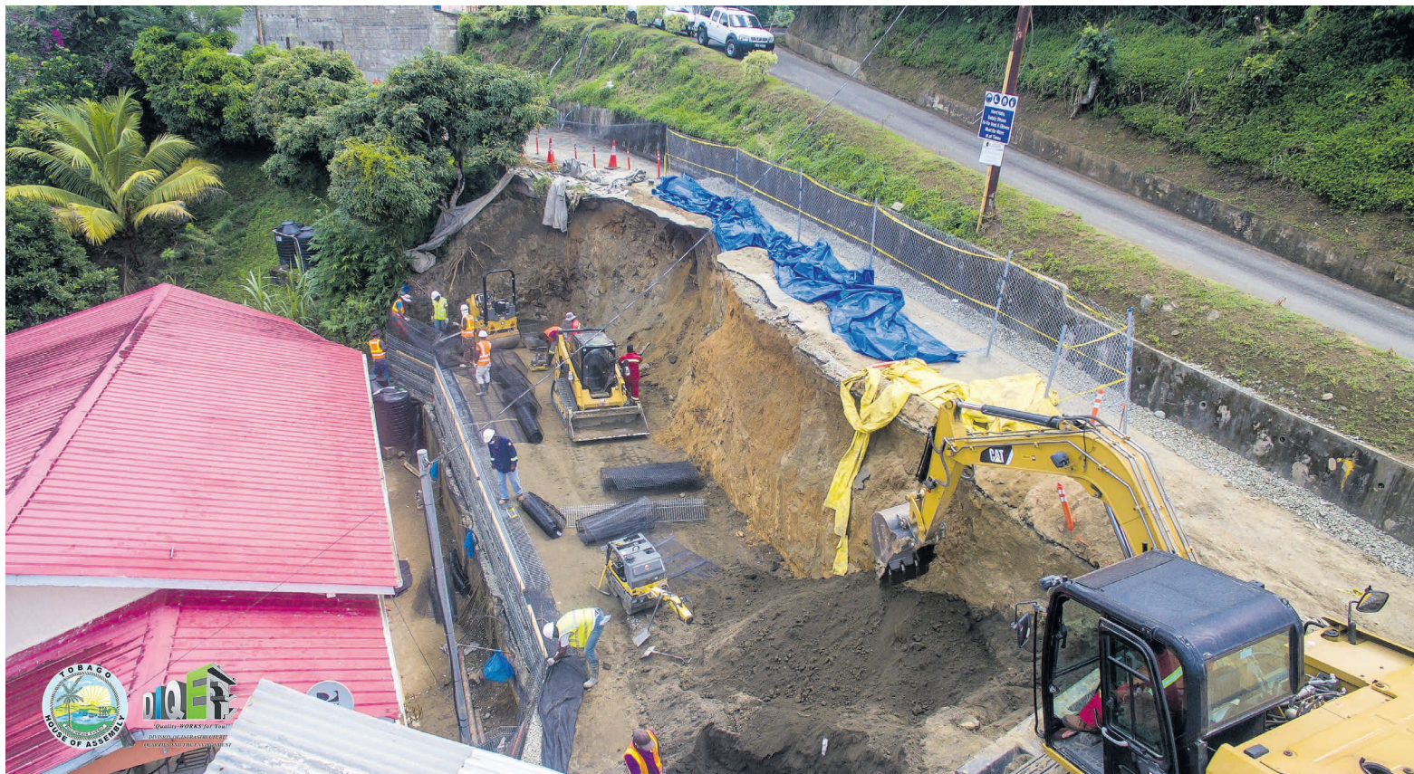
In this file photo, workmen build a retaining wall in Mason Hall, Tobago.
