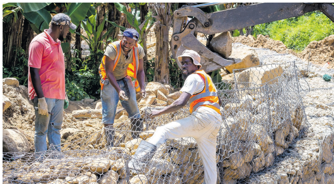
In this file photo, workers reinforce a river bank at Manswell Trace, Castara with a caged stone retaining wall.
