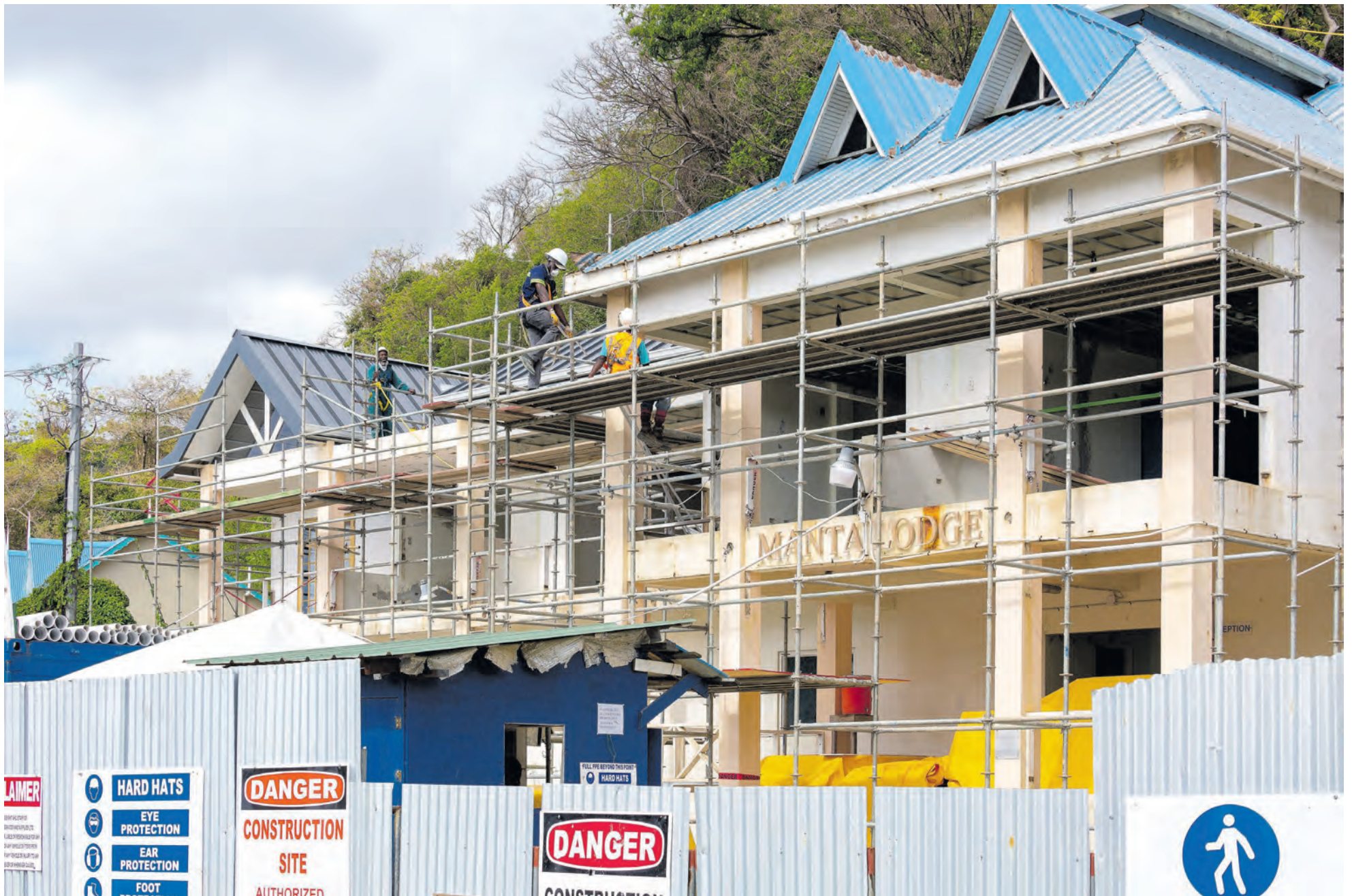
Construction workers at the Manta Lodge site in March 2021. PHOTOS BY DAVID REID
