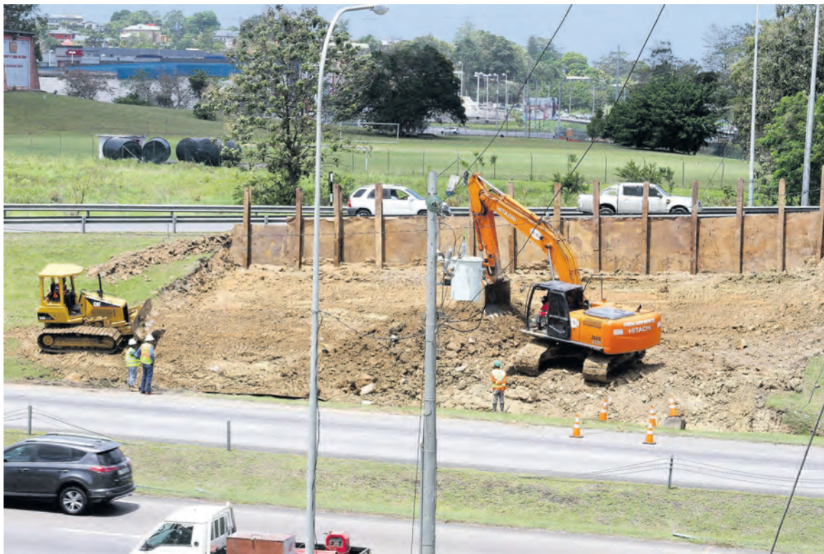
Ongoing works at the construction site of the Tarouba flyover. PHOTOS BY ANGELO MARCELLE
