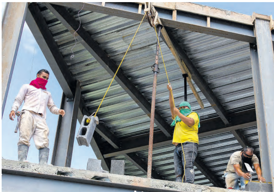
Workmen Nelson Ortiz, centre, Juan Serrano, left, and Junior Chirinos move concrete blocks to the top floor of a building on a construction site at Crooks River Road, Scarborough. PHOTO BY DAVID REID
