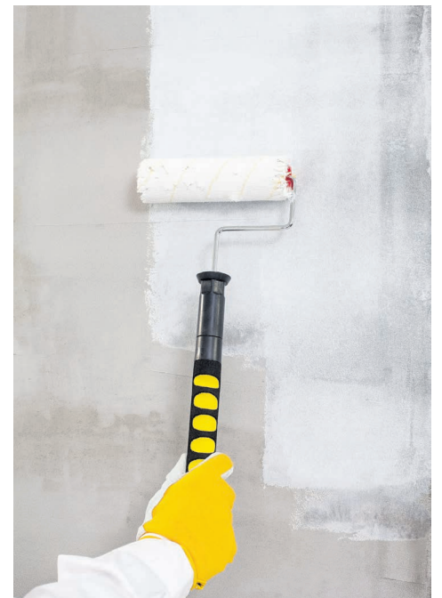
Prime freshly plastered walls before painting with your desired wall colour. PHOTO TAKEN FROM MODERNIZE.COM
