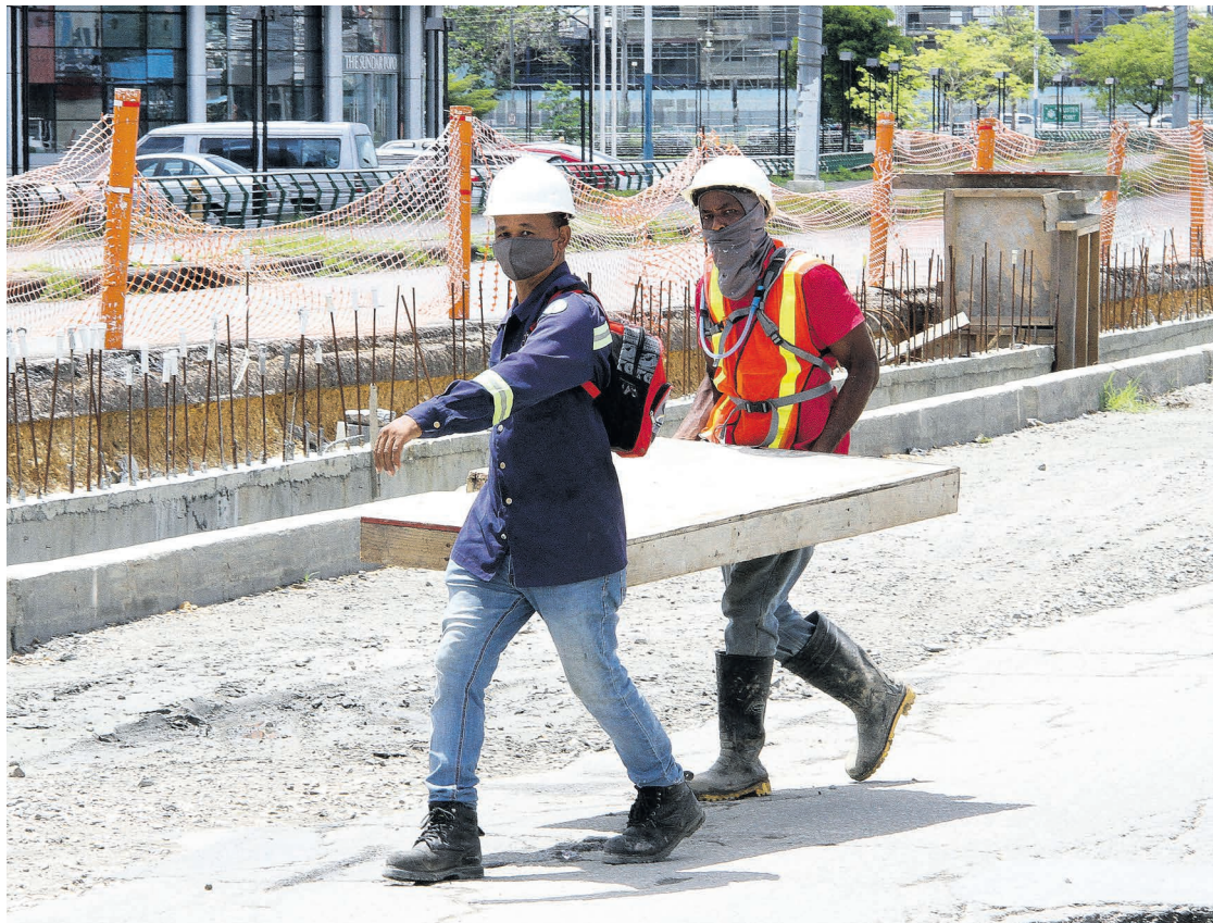
With the reopening of the construction sector, work on several public projects, including the San Fernando Waterfront project, has resumed. Public construction projects, like in many countries, are the backbone of government investment in the economy. PHOTO BY ANGELO MARCELLE
